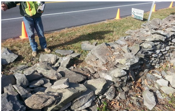
Stone wall work along Rte 9: Before (top); during repair by VEC and Adams Landscaping (bottom); and after completion, with NPS path (top of next column).
